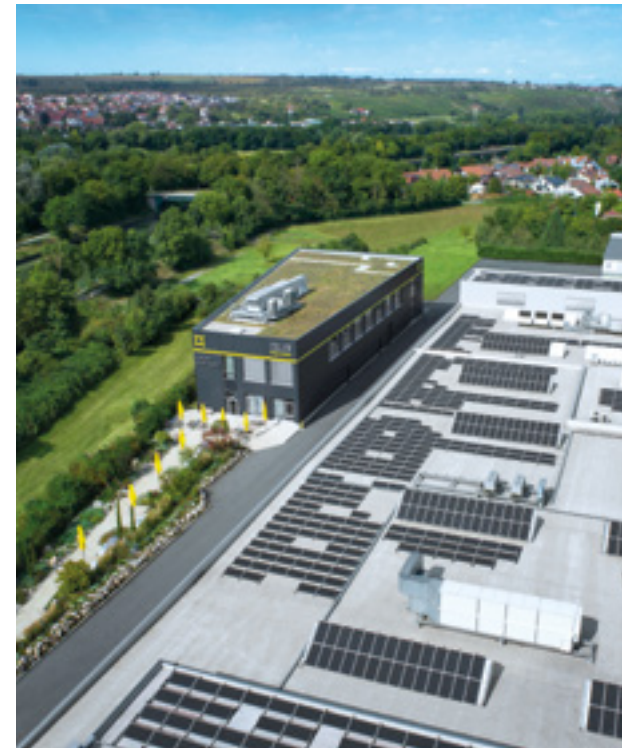
Solar panel system on the roof of the ZOLLER global headquarters
